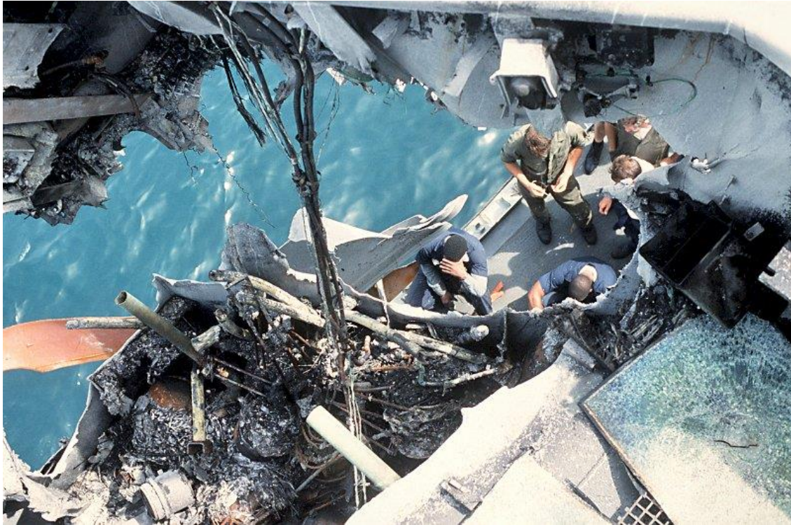
Above: Looking down to the main deck from the port bridge wing (01 level). Note that the explosion has completely blown the steel deck away. (Photo: Navsource.org)
